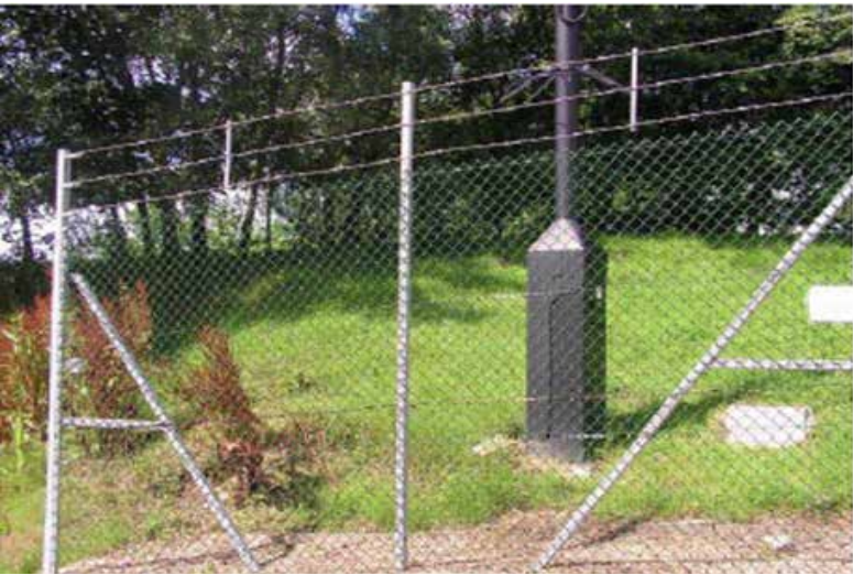
Figure 2: Class One Fencing
