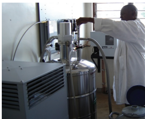
Liquid Nitrogen Plant that produces Liquid Nitrogen which keeps the vaccine in the required cool temperature for preservation
