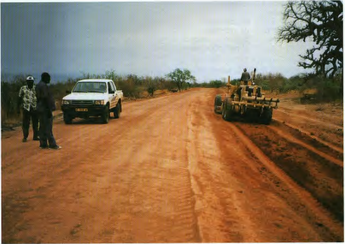
Bilango-Fada-Ngourma Road Project in Burkina Faso: opening up Gourma and Gnagna Provinces, and promoting regional economic integration with adjoining countries.
