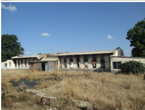
Fig 20: Paediatric ward building gutted by fire
