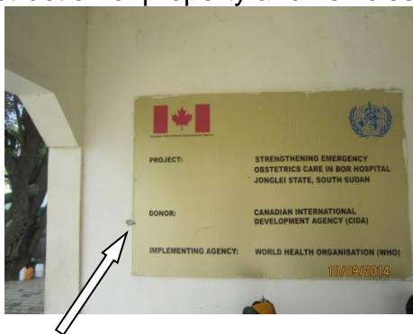
Fig 11 Bullet defect on hospital plaque At entrance to outpatient department
